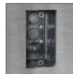
TA-62F Empty Junction Box
